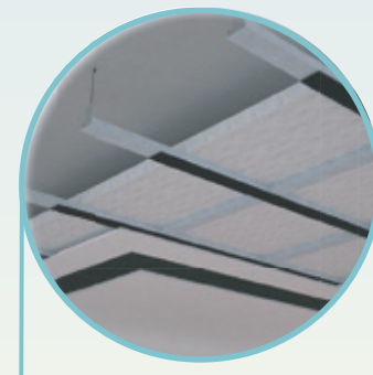
False ceiling insulation
